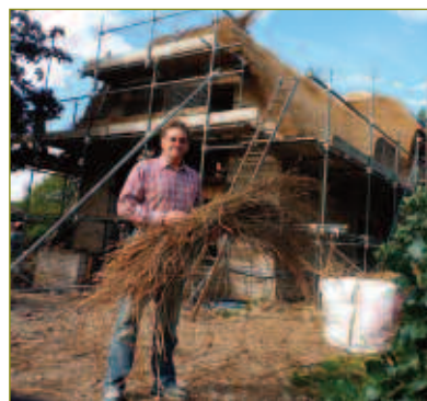
Above: Alvin is using Wicken sedge to thatch his roof. Below left: cutting and bundling in full swing
